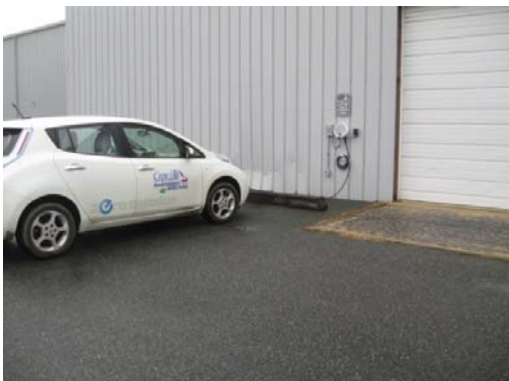
Photo 1: Three electric vehicle charging stations were installed at the airport for use by the public and airline tenants. Pictured here is Cape Air’s Nissan Leaf used for luggage concierge.
